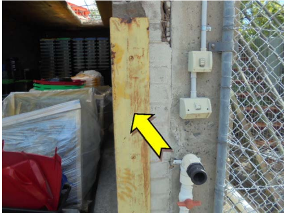
Photo Exterior, east elevation, metal framework – 1. suspected lead-containing yellow upper paint system.
